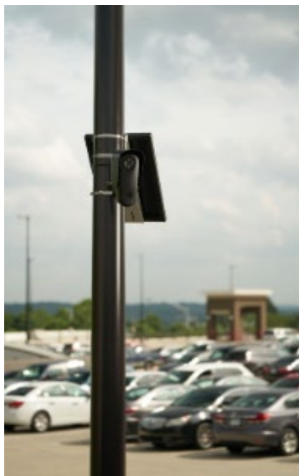
Solar & Existing Pole
